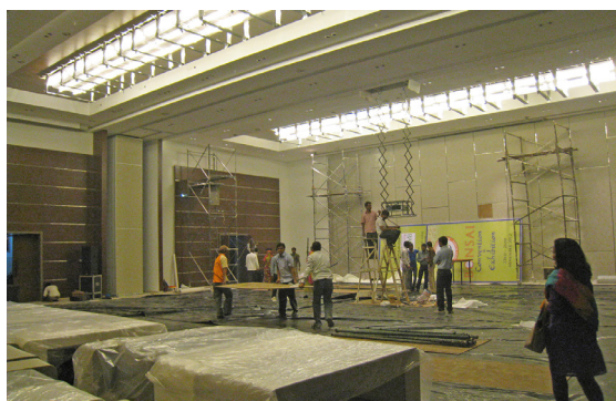
photos above! Now this is at 3:30 p.m. the day before the Opening Ceremony. Over 200 workers labored through the night to totally complete this building! They actually completed all the work around 2 a.m.
